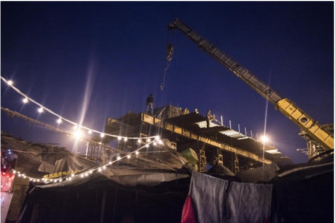
Even the temporary settlement is in danger of being evacuated since the Delhi Metro construction is getting intense in the area.
